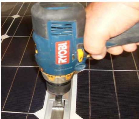
4. Using a 5/16" magnetic driver-drill screws into sheet metal until secure, check W/torque wrench to 30 to 36in-lbs.
